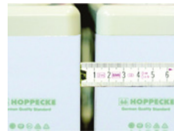
Fig. 5-14: 10 mm clearance between the batteries
